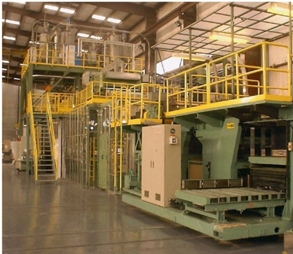
APET extrusion line 1 installed and operational on Jan 2012. APET extrusion line 2 is scheduled to be installed and begin production in 2014.
